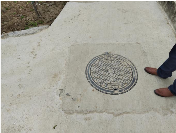
污水管检查井
